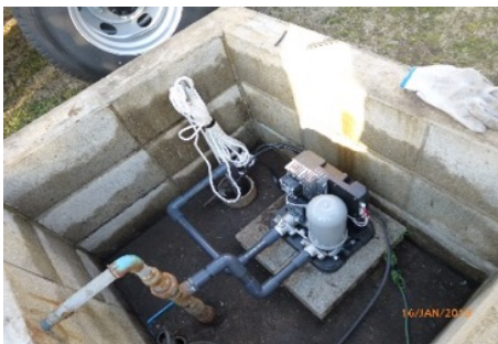
Figure 9. Revival of campus well for supply during disaster.
